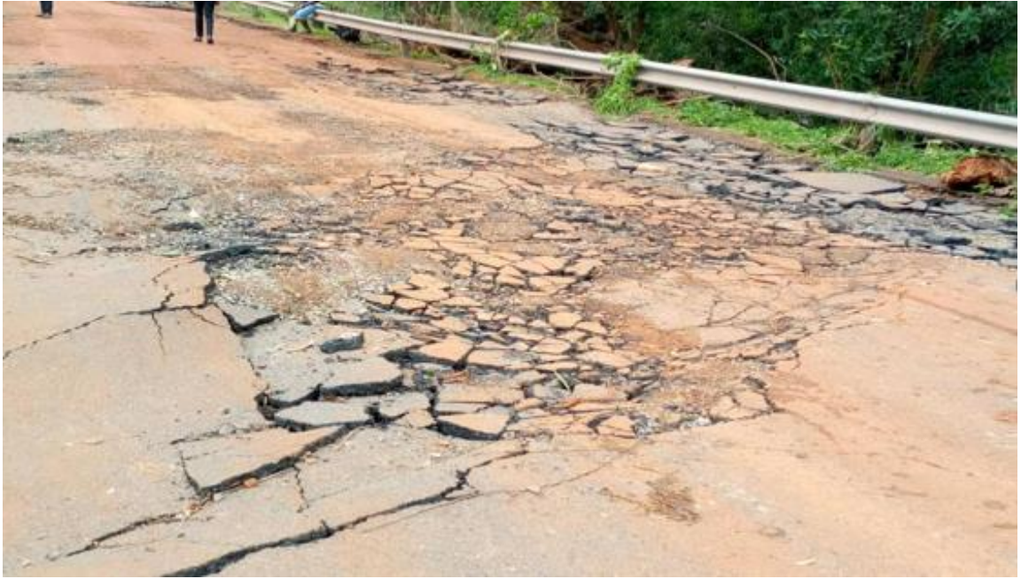
Figure 7: Destruction of roads
